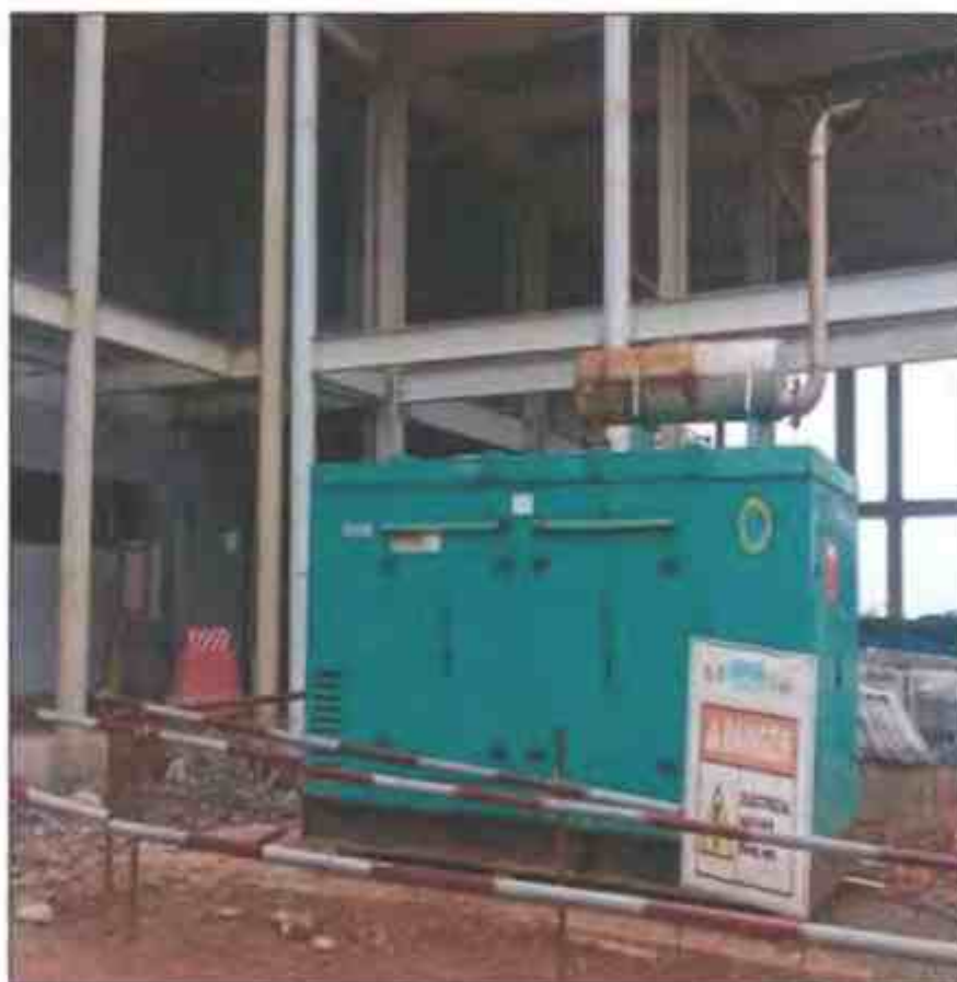
DG Set with adequate Stack Height
