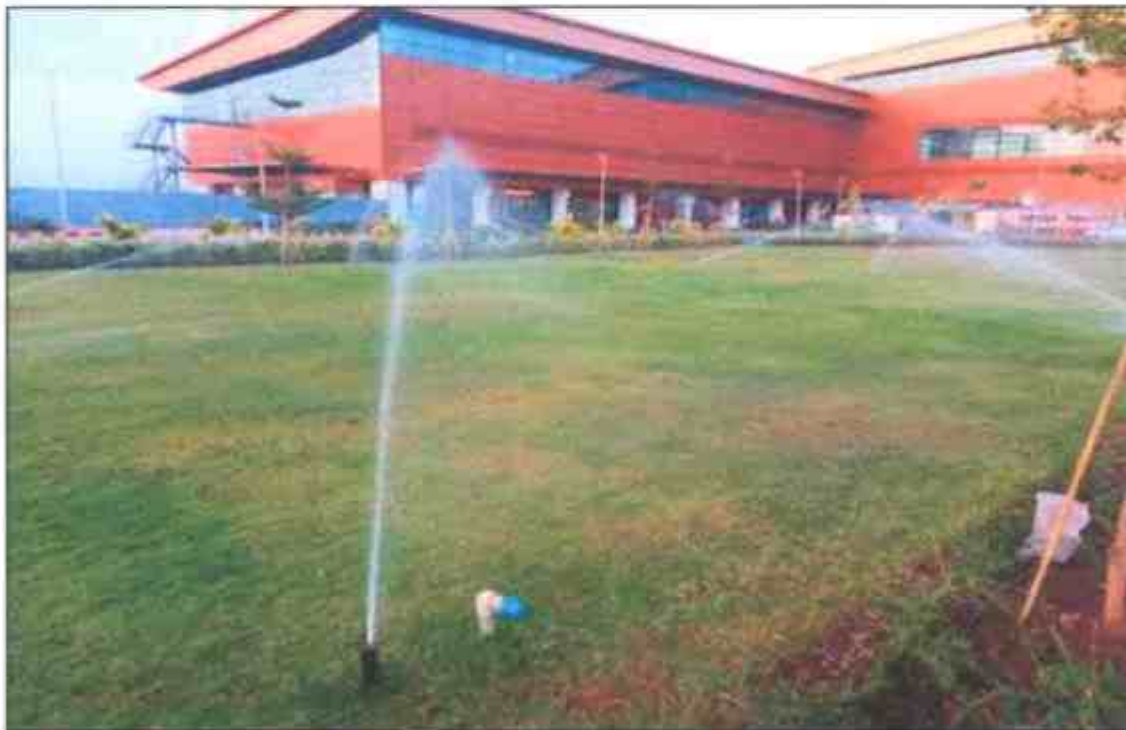
Sprinkler Irrigation for Landscaping & Avenue Plantation
